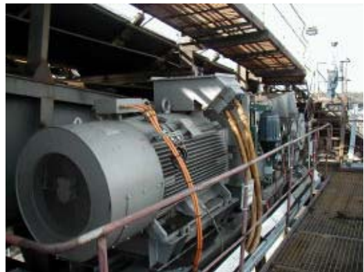
Figure 6: Conveyor Drive Motor
